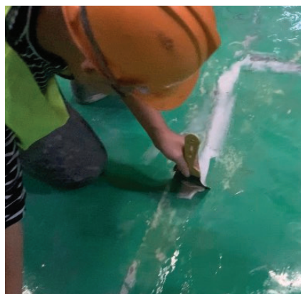
TRÁM THEO HÌNH CHỮ V Cut and widen cracks in the shape of "V"
